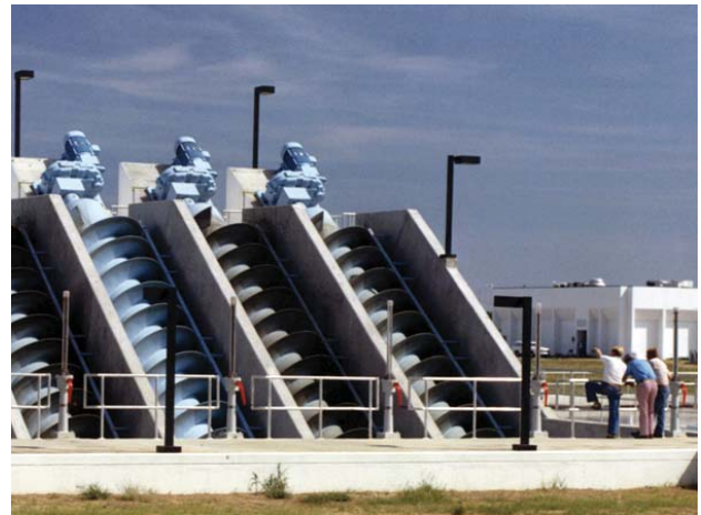
Archimedes screws pump wastewater in a treatment plant in Memphis, Tennessee, USA. Each of these screws is 96 inches (2.44 meters) in diameter and can lift 19,900 gallons per minute. Manufactured by Lakeside Equipment Company of Bartlett, Illinois, USA.
